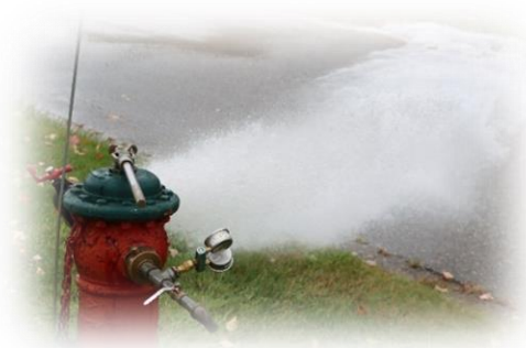
During a flushing operation you'll see crews flushing via fire hydrants and end of water main blow off pipes.
